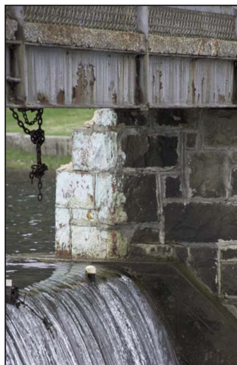
Photo by Toan Mach Cold Stream Dam, in Philipsburg, was constructed in 1889.
