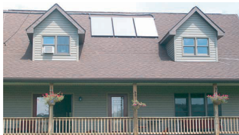
Solar Hot Water System
