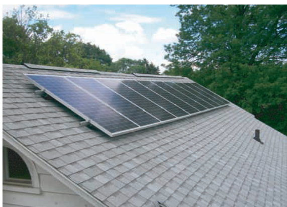
Solar Electric System
